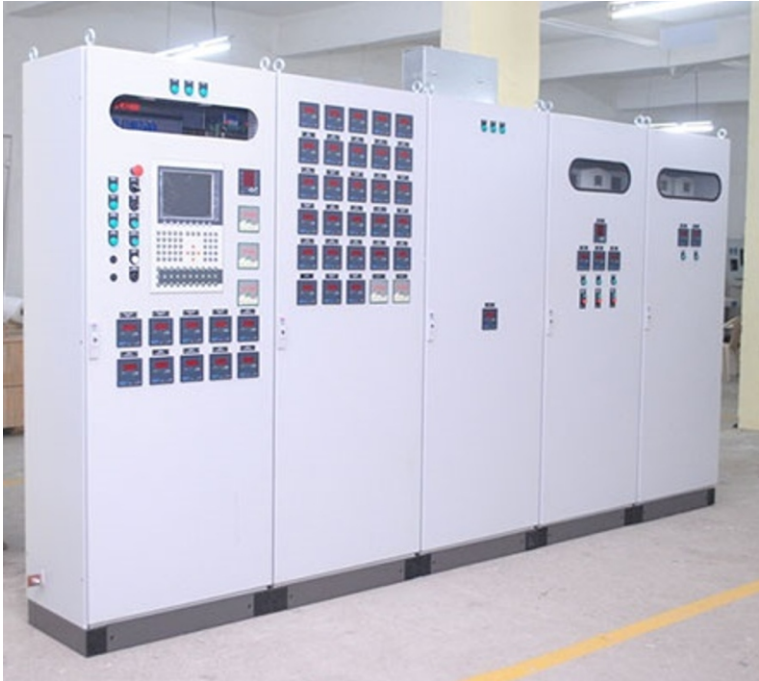
CE Certified PLC Controlled VFD Panel Client : Jagmohan Pla-Mach Pvt. Ltd.
